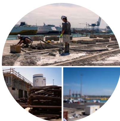
SEINGIM ELECTRIFICATION OF NINE BERTHS, PORT OF CIVITAVECCHIA, ITALY
